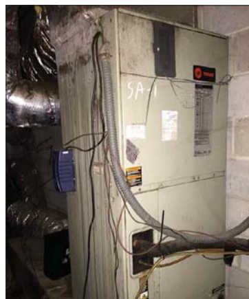
Existing HVAC Equipment
