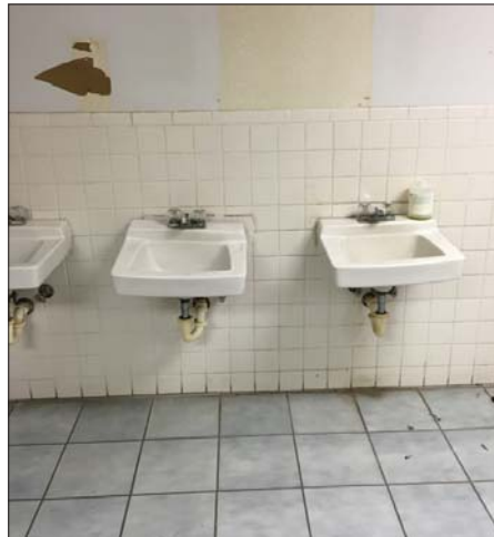
Water Damage At Sinks
