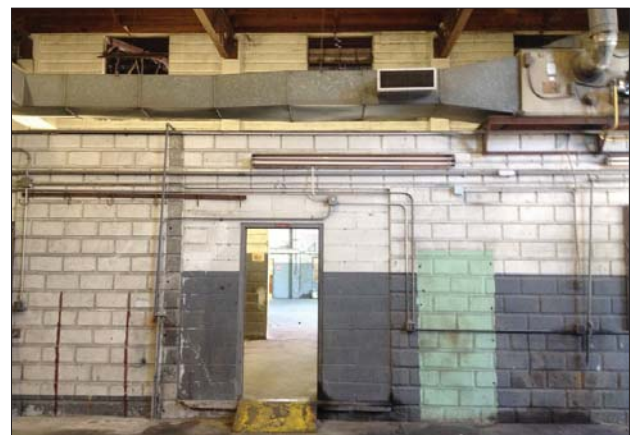
Maintenance Bay with Ductwork
