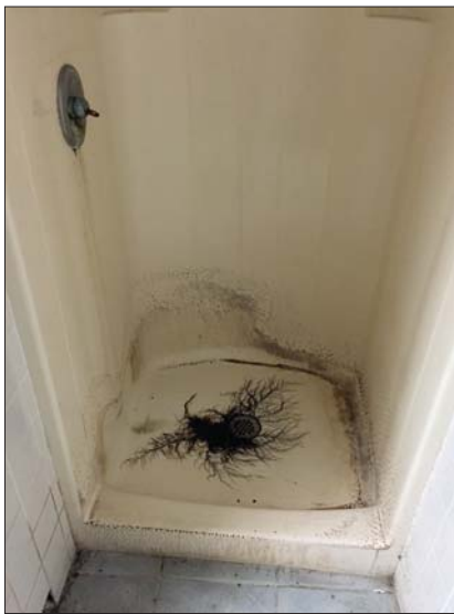
Extreme Mold Growth In Locker Room Shower
