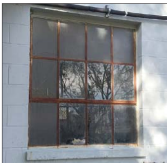
Rusting Window Panes
