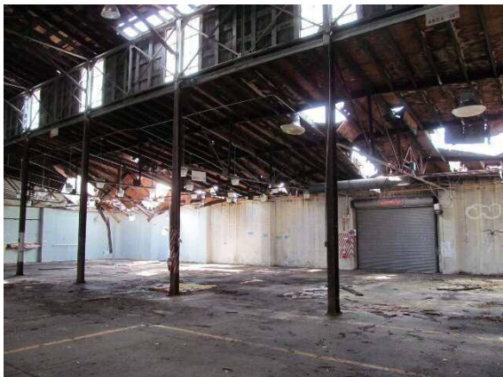
Warehouse area ceiling damage
