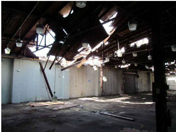
Warehouse area ceiling damage
