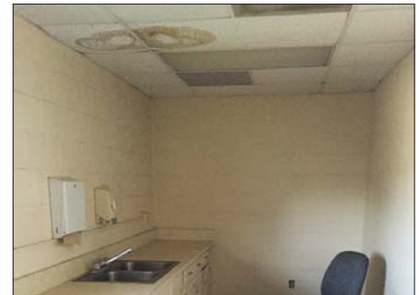
Water Damaged Ceiling Tiles
