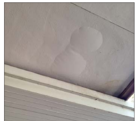
Damage Indicating Possible Roof Leak
