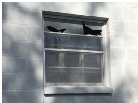
Broken Window Glass
