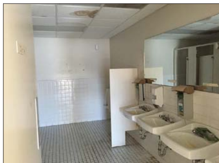
Dilapidated Toilet Room
