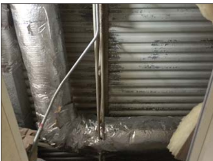
Ductwork Above Ceiling
