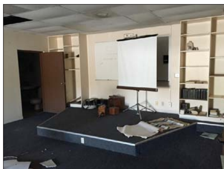
Sagging Ceiling Tiles And Worn Carpet
