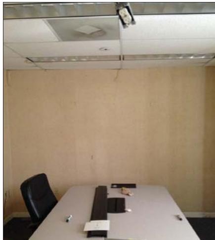
Electrical Components Hanging From Ceiling
