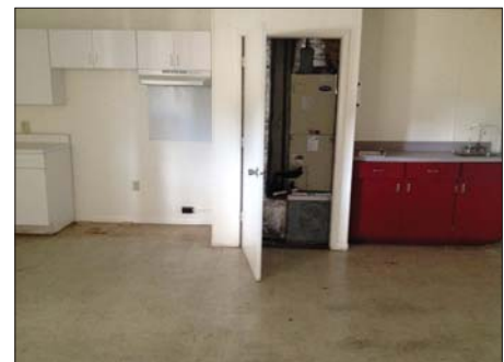
Mechanical Closet In Break Room
