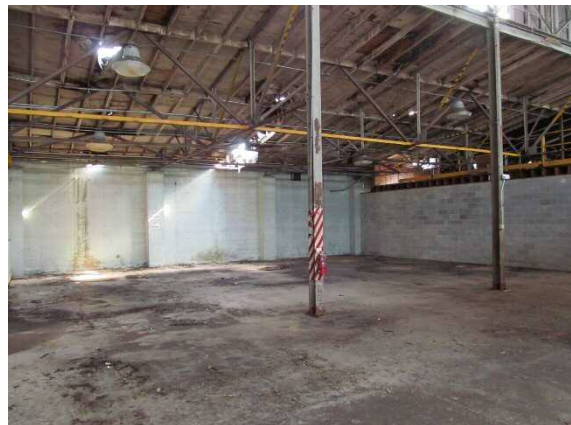
Warehouse area ceiling damage
