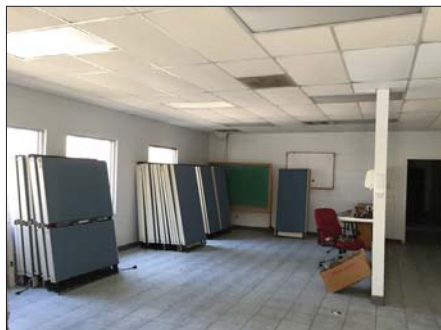
Office With Sagging Ceiling Tile
