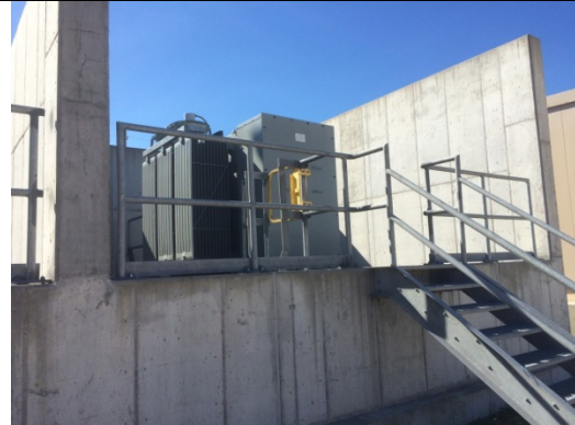
Detail: Area Transformers
