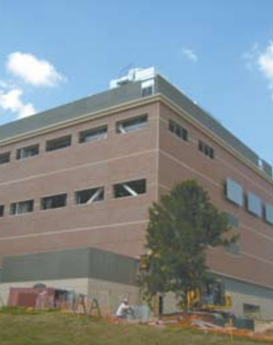
GRU's South Energy Center is scheduled for completion in February 2009.
